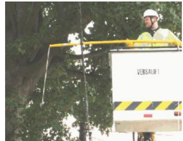
EPT/OHP/B011 - Overhead Distribution
