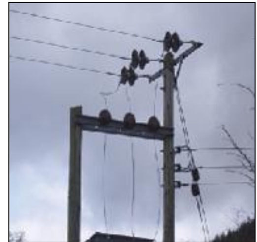
33kV HIGH voltage AND LOW voltage line on the same pole
